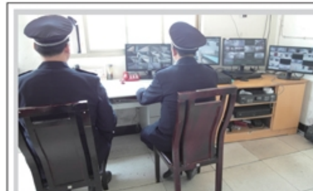
Security Monitoring & Controlling System 门卫及安全监控系统
